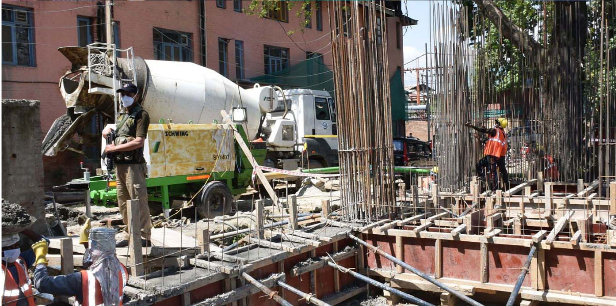
Dr Syed Abid Rasheed Shah inspected progress on construction of 120 bedded Specialized Orthopaedic Unit. Source: DIPR
